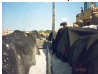
Active Gas Extraction System Fredericksburg, VA
