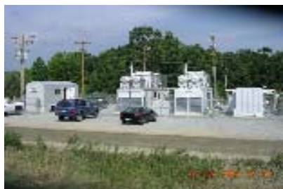
Landfill Gas to Energy
