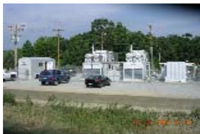
Landfill Gas to Energy
